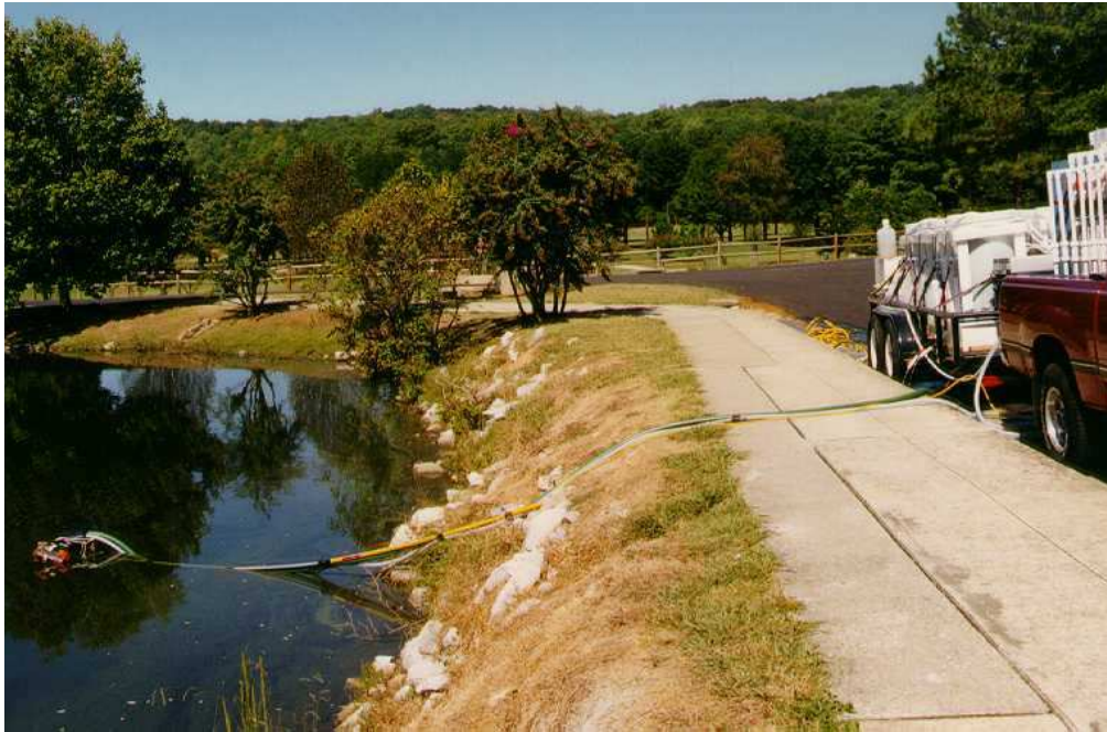
Figure 3. The set-up for the pilot-scale tests showing the pumps in the lake, sending water up to the manifold for distribution into the individual filters.
