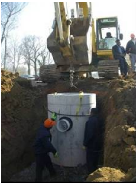
Figure 3. Installation of Tuscaloosa UpFlo™ filter.
