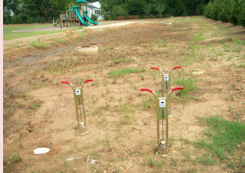
Very little "bio" in this biofilter, indicating compacted media having adverse affects on plant growth.
