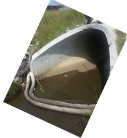
Hydrodynamic Device Outlet/ Dry Pond Inlet
