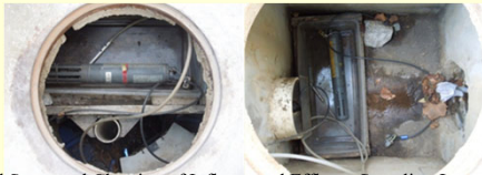
Pre-Storm Field Setup and Cleaning of Influent and Effluent Sampling Locations Showing Sampling Trays for Cascading Flows
