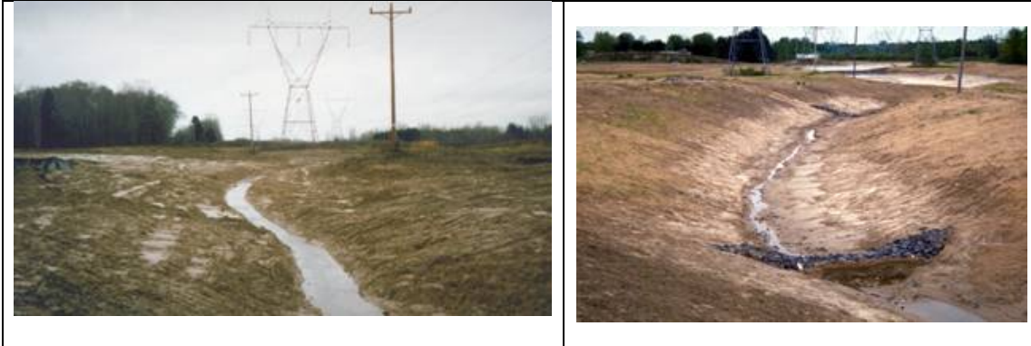
This exposed site is under a state shutdown order for destroying 2 acres of walleye spawning area in a nearby lake. 65 acres of the 70 acre site was stripped exposing soil containing 75 – 98 percent fines that could not settle out on site.
