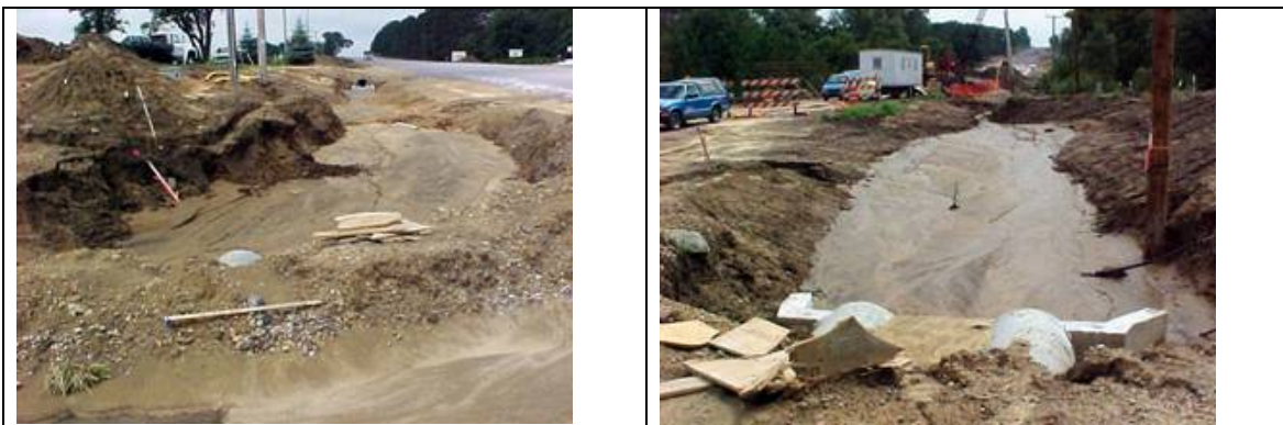
Drainage Filled with Construction Sediment (J. Voorhees)
