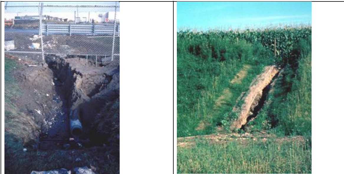
Poor Drainage Construction
