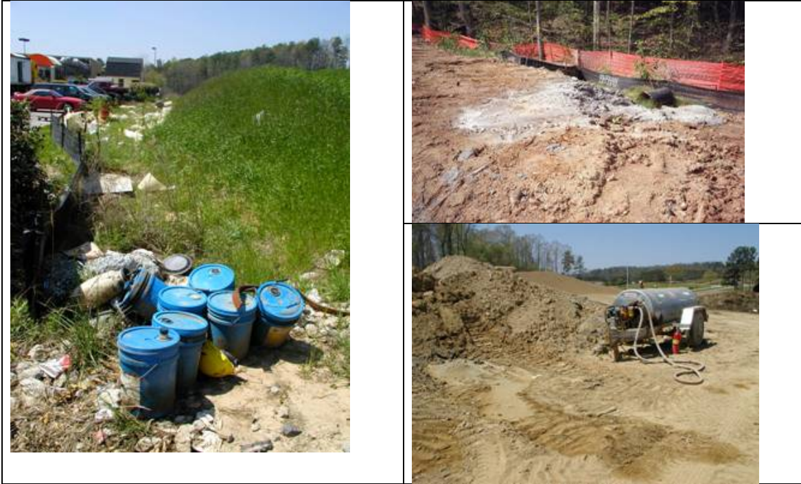
Improper Disposal of Construction Debris and Improper Equipment Maintenance
