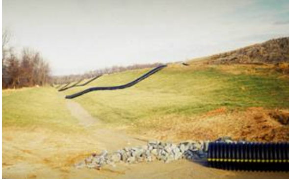
This photo of U.S. Route 1 being relocated around Dover, Delaware shows pipe slope drains that carry sediment laden runoff downslope to a collector swale. Note that the side slopes are graded and seeded as the work progresses to keep soil from washing down.
