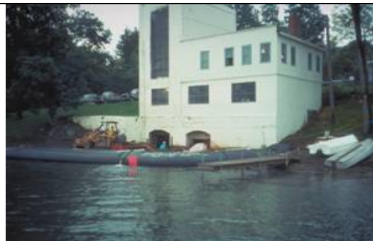
These two photos at the New York State Electric & Gas Corporation hydro-electric plant on Keuka Lake demonstrate the use of water structures as cofferdams. Two tubes of polyethylene wrapped with a geo-textile, these are filled with water to
