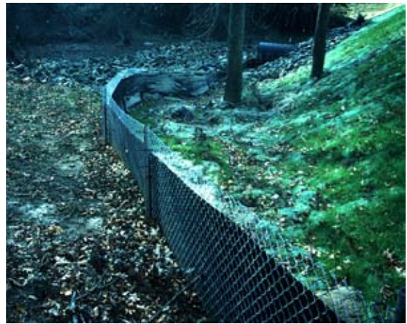
Super silt fence
