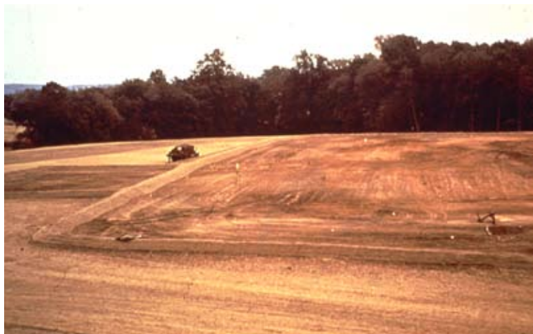
Example of an earth dike flow diversion
