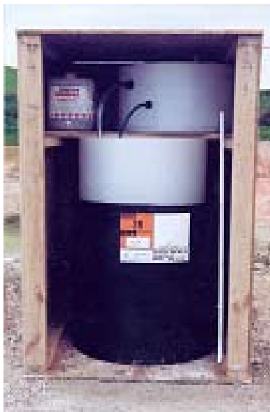
Example of an on-site chemical flocculation system
