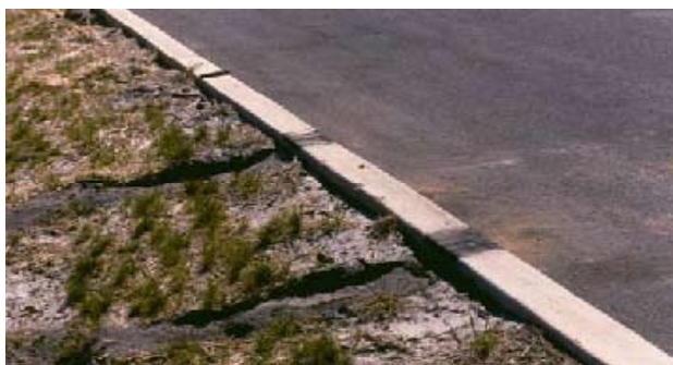
BAD: Lack of depressed curb hinders access to practice by maintenance personnel and equipment.
