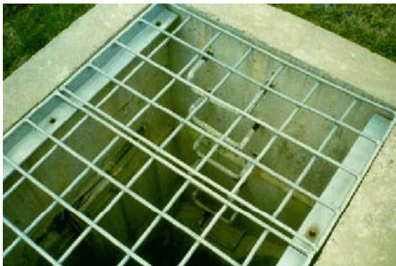
GOOD AND BAD: Ladder rungs allow access to structure bottom, but large grating openings are hazardous to maintenance personnel.
