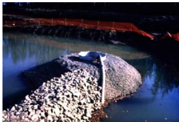
Sediment dewatering pit
