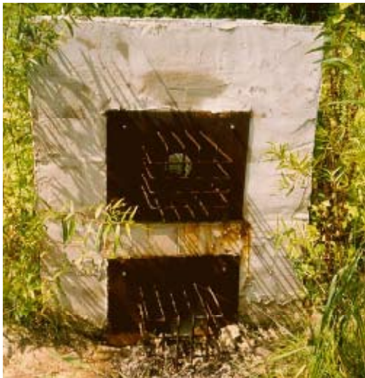
BAD: Inappropriate materials and poor construction increases maintenance effort and cost.
