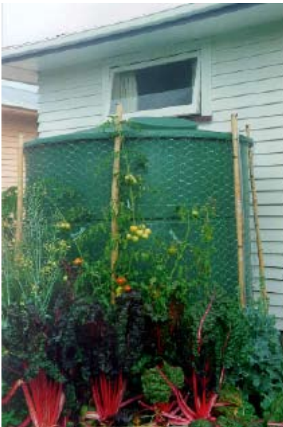
Water tank capturing roof runoff
