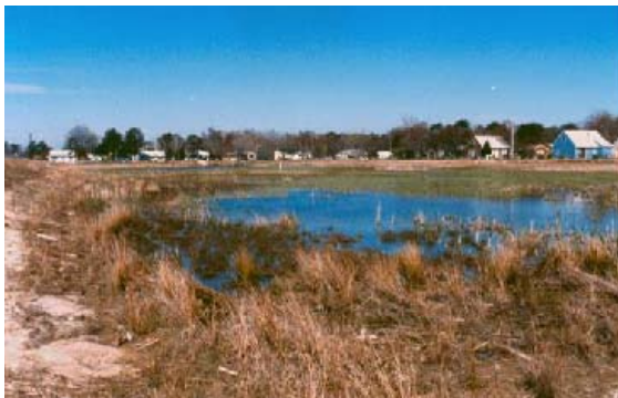
BAD: Lack of adequate bottom slope in dry detention basin causes unintended ponding that prevents mowing and cleaning.
