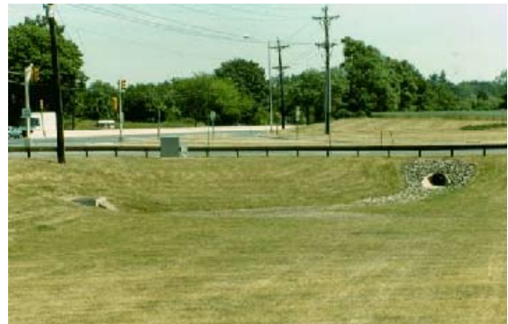
GOOD: Adequate bottom slope in dry detention basin creates intended dry bottom that can be regularly mowed and cleaned.
