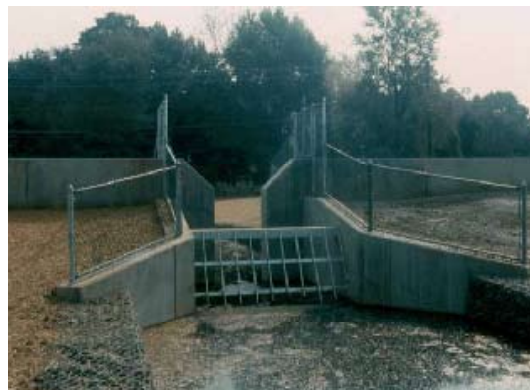
To help ensure sound construction, required construction materials and procedures should be as standard as practical. Unique procedures and complex components should be thoroughly described and detailed in construction documents.
