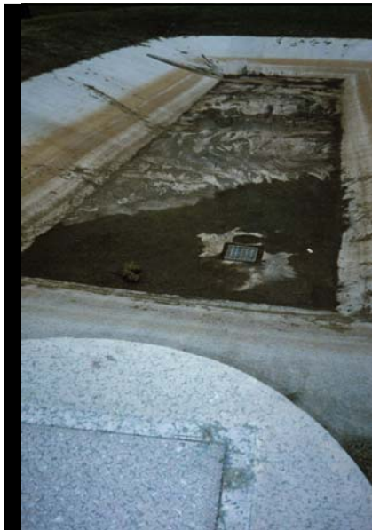
Dry Pond to Equalize Flows before Sand Filter, Austin, TX
