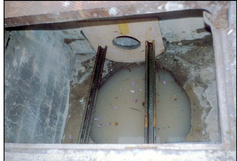
Retro-fitted Catchbasin with Sump Tested at Ocean County, NJ
