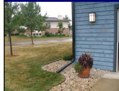
Disconnected roof drain
