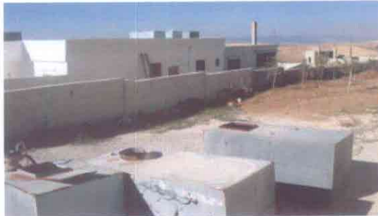
Old water tanks (1m 3 and 2 m 3 ) on the ground in Jordan, with newer tanks on top of the house. Photo by Laith Al-Faqih
