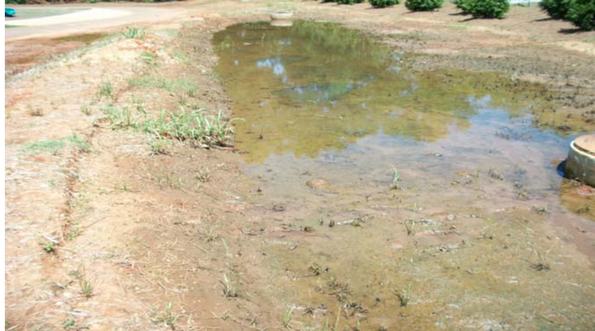
Figure3. Ponded water on the biofilter surface observed after rainfall events and double ring infiltration measurement installations.
