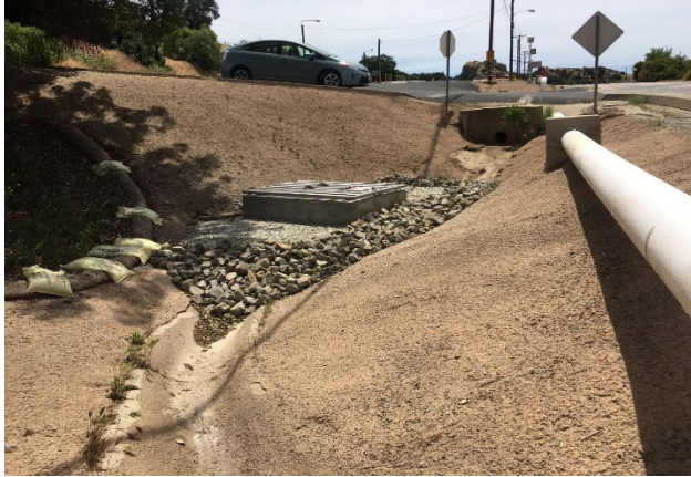
Figure 6. Upper Parking Lot Media Filter
