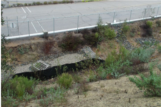
Figure 3. B-1 Sedimentation Basin and Media Filter
