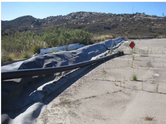
Figure 9. Berms and pumps at helipad used to divert flows to Silvernale stormwater treatment system began in 2011.
