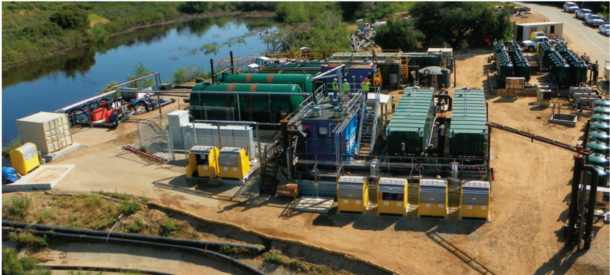
Figure 8. Outfall 018 Silvernale stormwater treatment system and adjacent storage pond completed in 2011.
