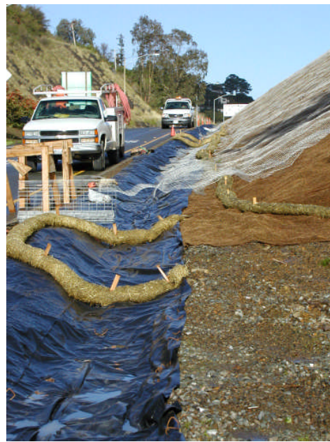
Plastic tarp, with coir logs, for a temporary liner and to slow the velocity.
