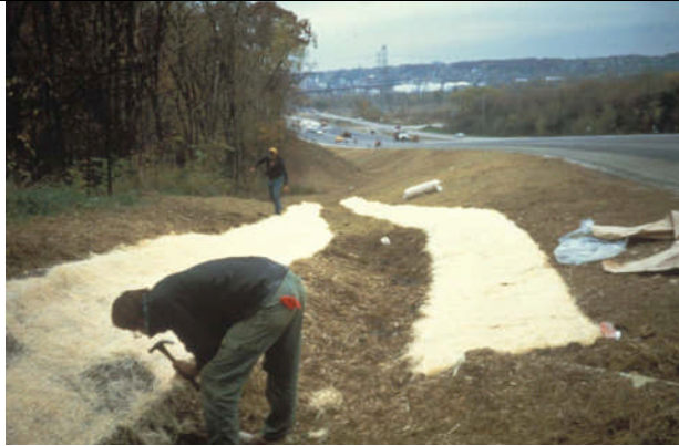
Installation of reinforced liner along thalweg of channel, with other material along sides (VA photo).
