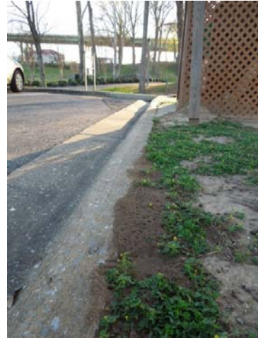
Fire ant hills besides the filter inlet increased the sediment load into the filter during some storms due to erosion
