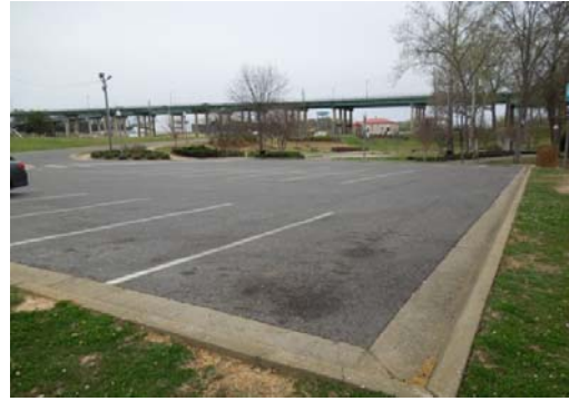
Asphalt pavement with oil and grease stains
