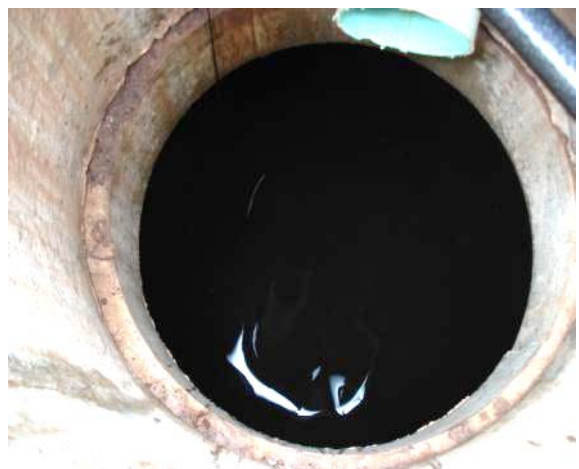
Dry well with standing water (9 Fox Hill)
