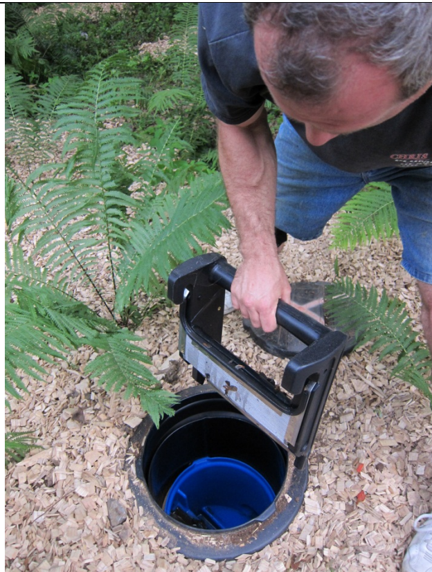
Cistern inlet filter.
