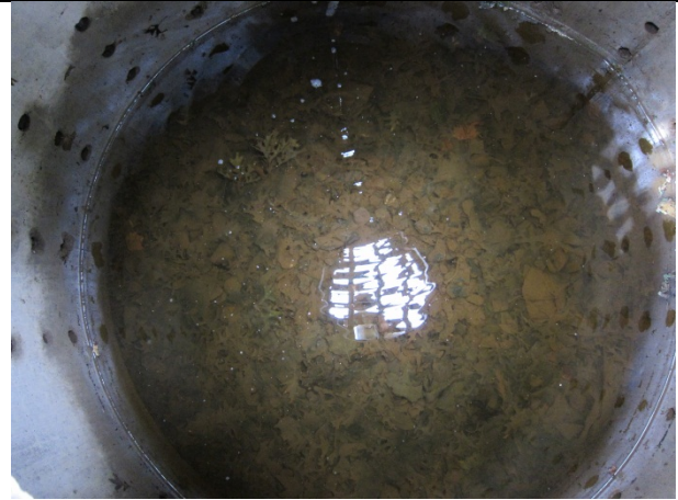
Dry well with standing water and some leaves.
