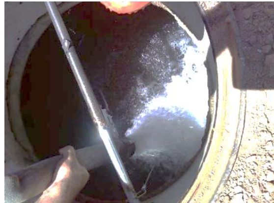
Dry well with standing water (1 Sinclair Terrace)
