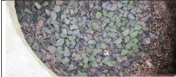
Dry well showing crushed stones at bottom with some minor lawn debris.
