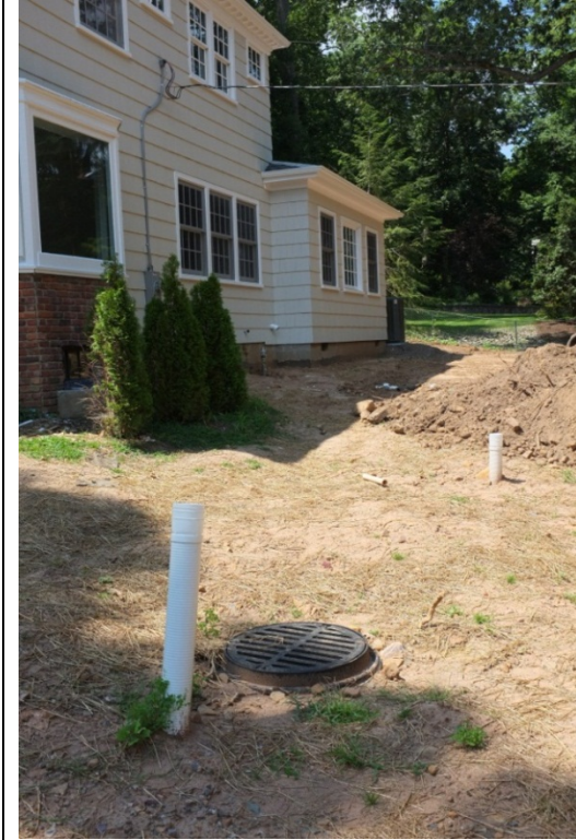
Frontyard dry well at new home used for water quality monitoring on Slope Drive open grating receives surface inflows in addition to roof runoff.
