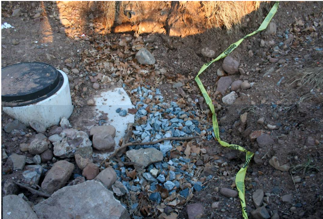
Figure 2-3. Installed dry well in Millburn, NJ, showing the surrounding blanket of crushed stone before completion of the backfilling (photo from Mel Singer).
