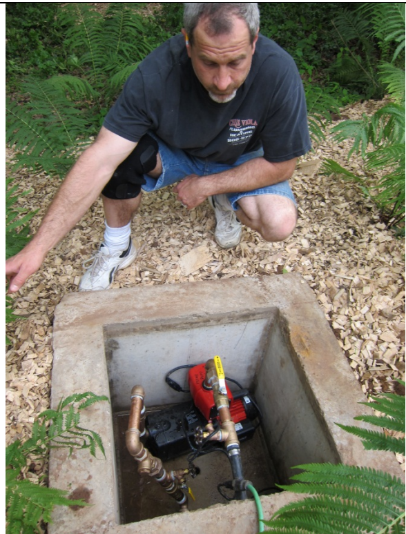
Cistern irrigation pump.
