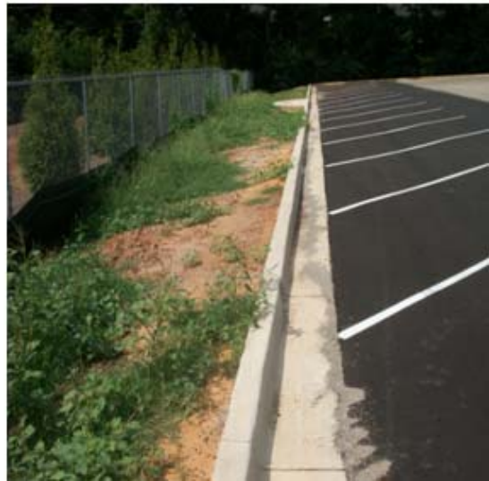
Parking lot edge and eroding soil
