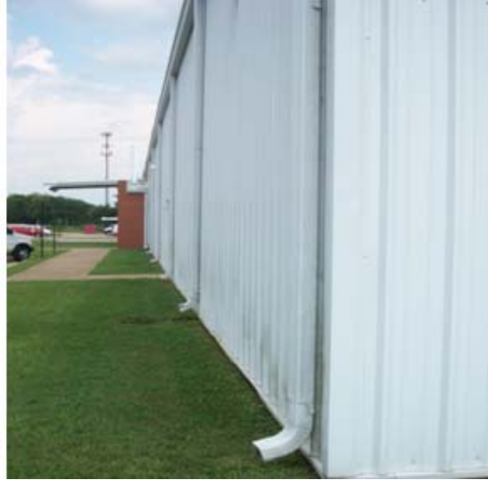
Disconnected roof from painted galvanized steel building draining to turf area.
