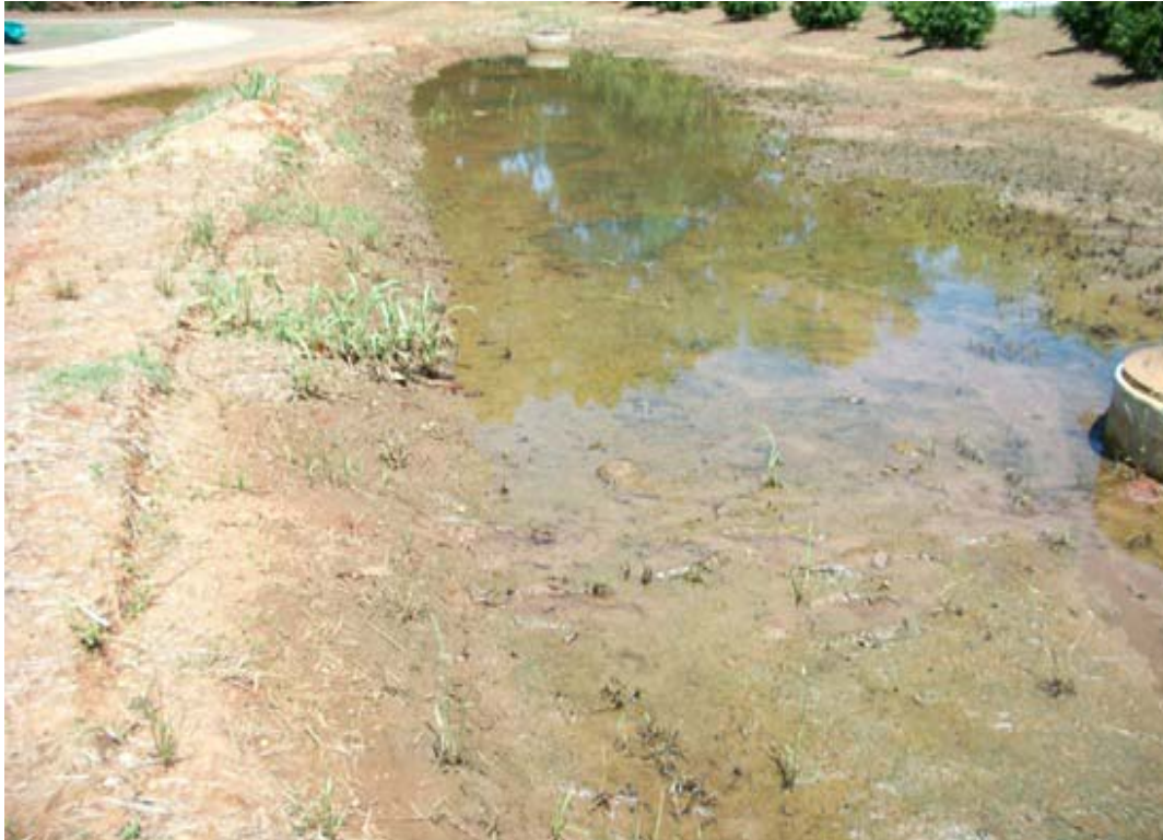
Figure 65. Poned Water on the Biofilter Surface Observed after Rainfall Event. (The Vegetation Cover Is Very Poor Indicating Likely Serious Compaction).
