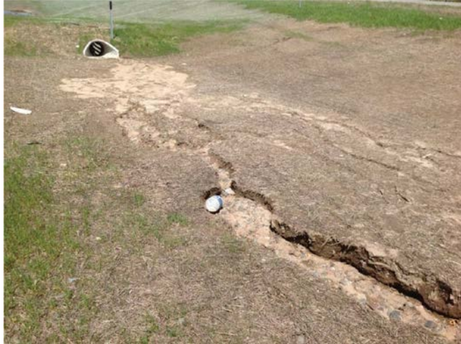
Figure 18. Erosion of side slopes and basin floor in Pine Bend infiltration basin.
