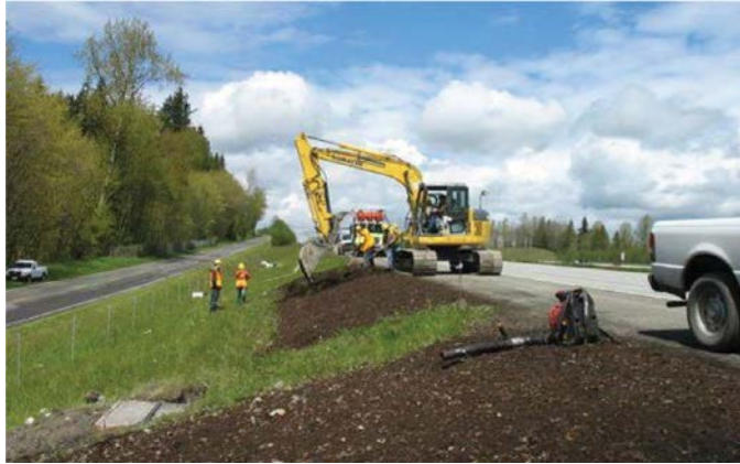
Figure 21. Construction of I-5 Pilchuck vegetated filter strips. Photo illustrates installation of compost amended vegetated filter strips (CAVFS) and modified vegetated filter strips (VFS). (Photo provided by Fred Bergdolt, WSDOT.)
