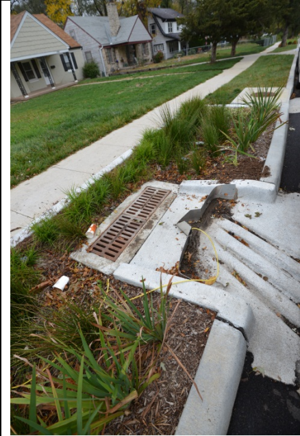
No samplers, but 2 level recorders at inlet and bottom of rain garden
