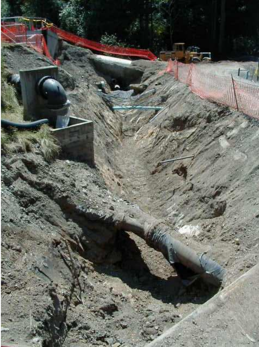
Photo 5-6. Photo of where the 277,200 gallon gasoline leak occurred (copyright 1999 nwcitizen.com. Reprinted with permission).
