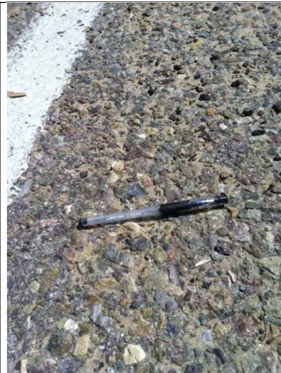
Photo 18: Parking lot near bldg 599- Very rough asphalt- Mixed Use Area
