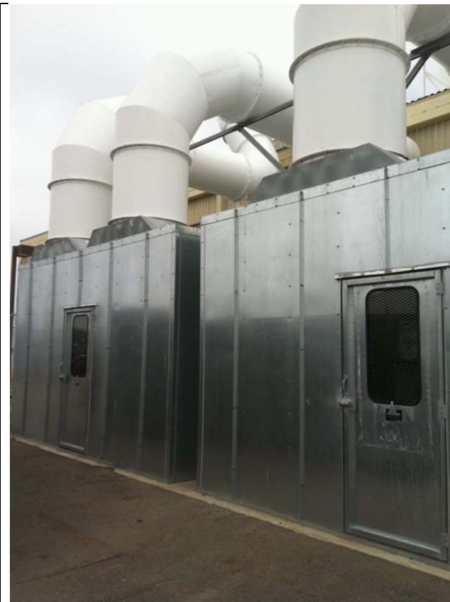
Photo 14: Metal scrubber vault to capture paint fumes and particles
