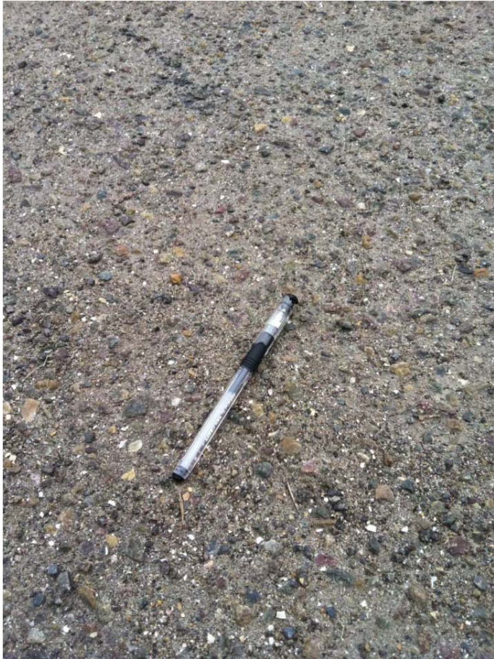
Photo 2: Rough asphalt roadway
