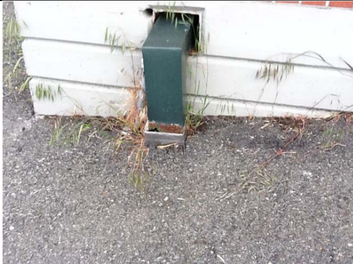
Directly connected roof drain. Drainage rear of Bldg. 2202 representative of entire 2200/2202 complex.
