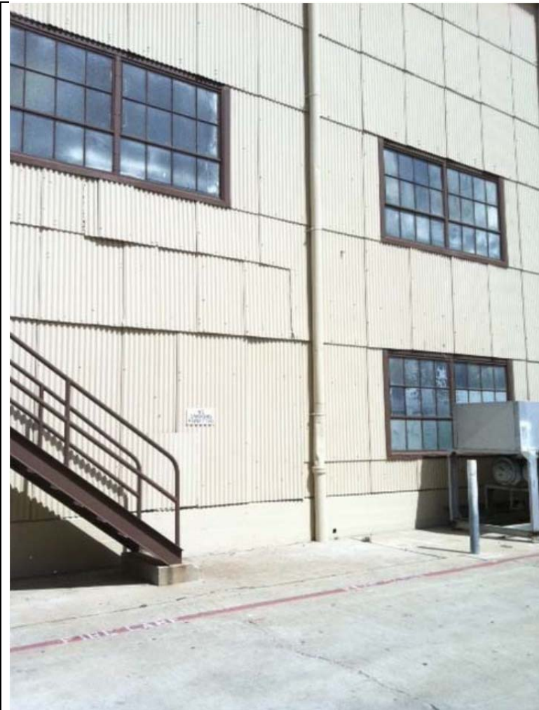
Photo 5: Building 94 runoff directly connected- Industrial North
