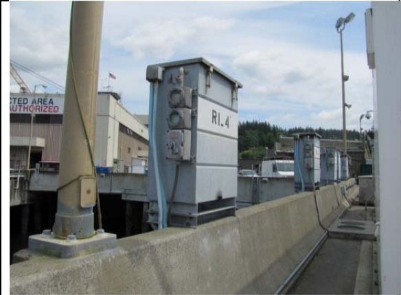
Other galvanized material areas (other impervious area #10). Photo 8: Galvanized utility box, 40 boxes on site.
