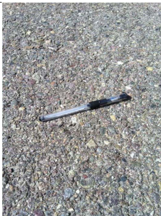
Photo 16: Rough asphalt around Bldg 461- Industrial Southeast
