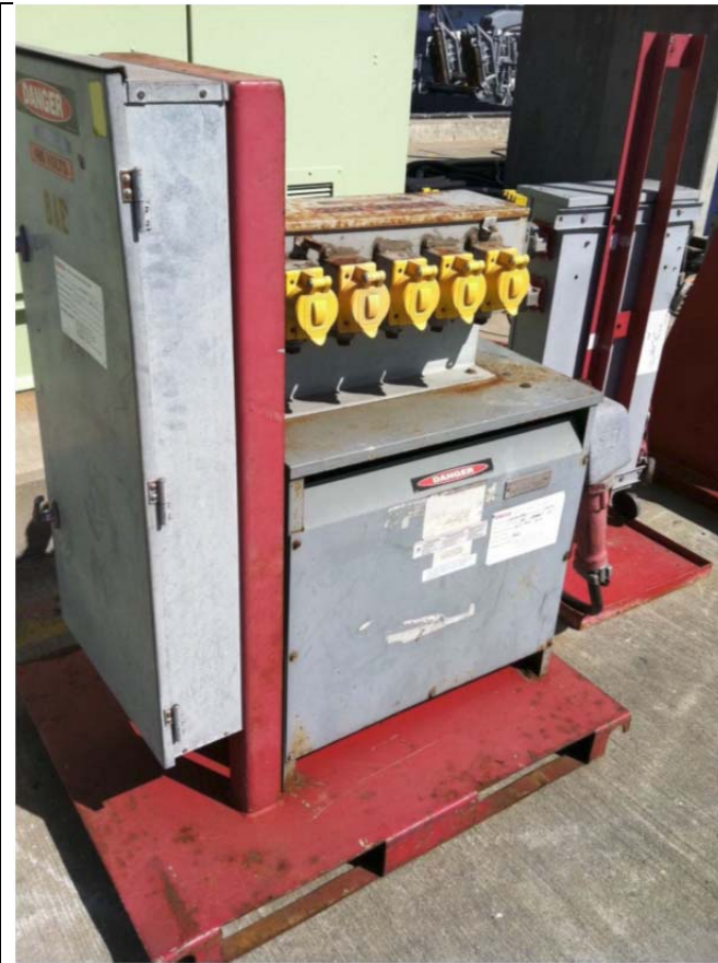
Photo 2: Galvanized utility box
