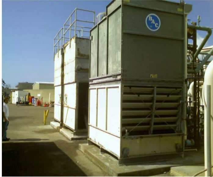
Photo 15: BAC A/C Chiller Units- Industrial Southeast
