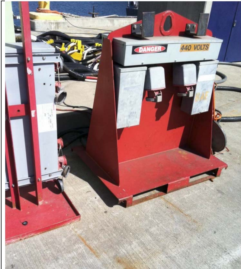
Photo 1: Galvanized circuit breaker boxes
