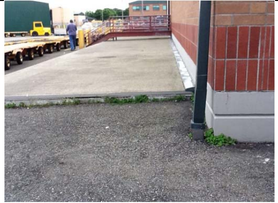
Directly connected roof drain. Rear Bldg. 2202 showing concrete pad, directly connected drainage and painted galvanized walkway/stairs.
