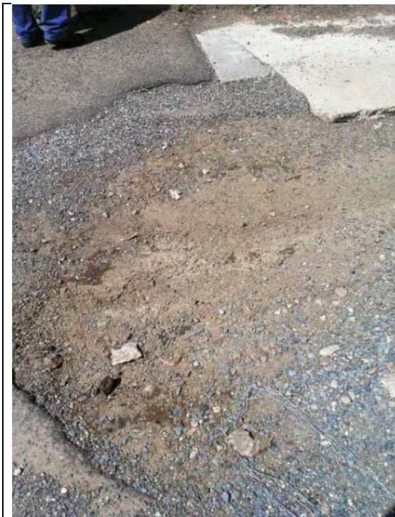
Photo 3: Very rough, degraded asphalt- Industrial North
