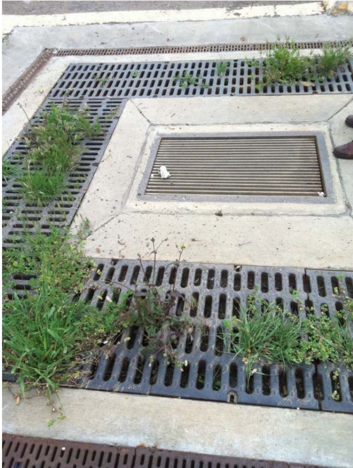
Photo 11: Catchment basin that conveys stormwater to Outfall 9
