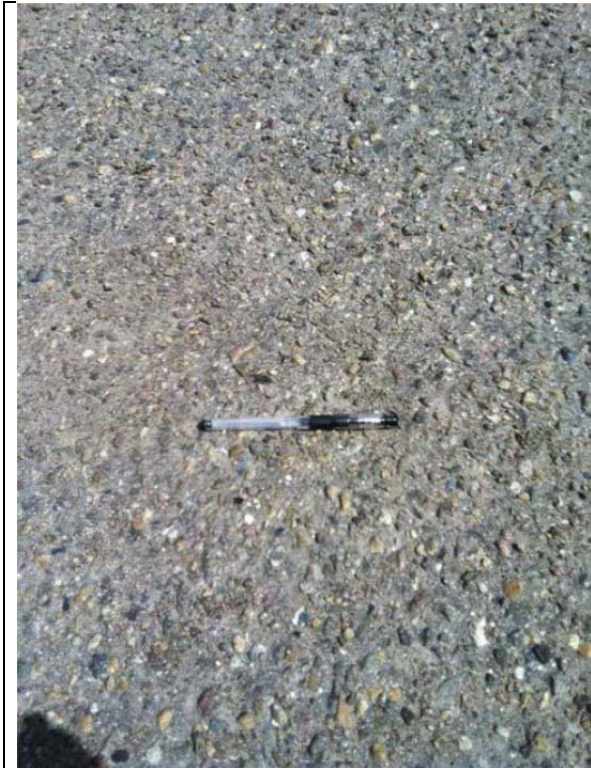
Photo 6: Rough asphalt around building 399- Industrial West
