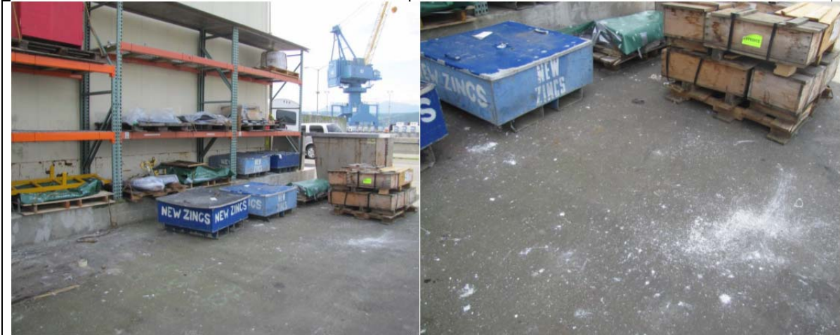
Other galvanized material areas (other impervious area #10). Photo 20: Storage and laydown including zinc anodes. Note corroded anode material on ground.
