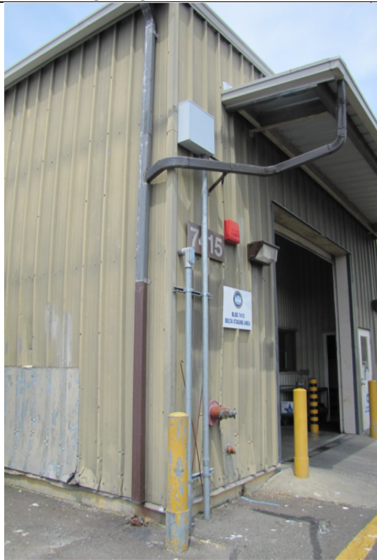
Galvanized metal roofs (other impervious area #9). Photo 5: Building 7414, painted galvanized w/significant paint peeling of wall. Note broken drainage, connected.
