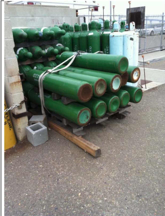
Photo 3: Gas cylinder storage
