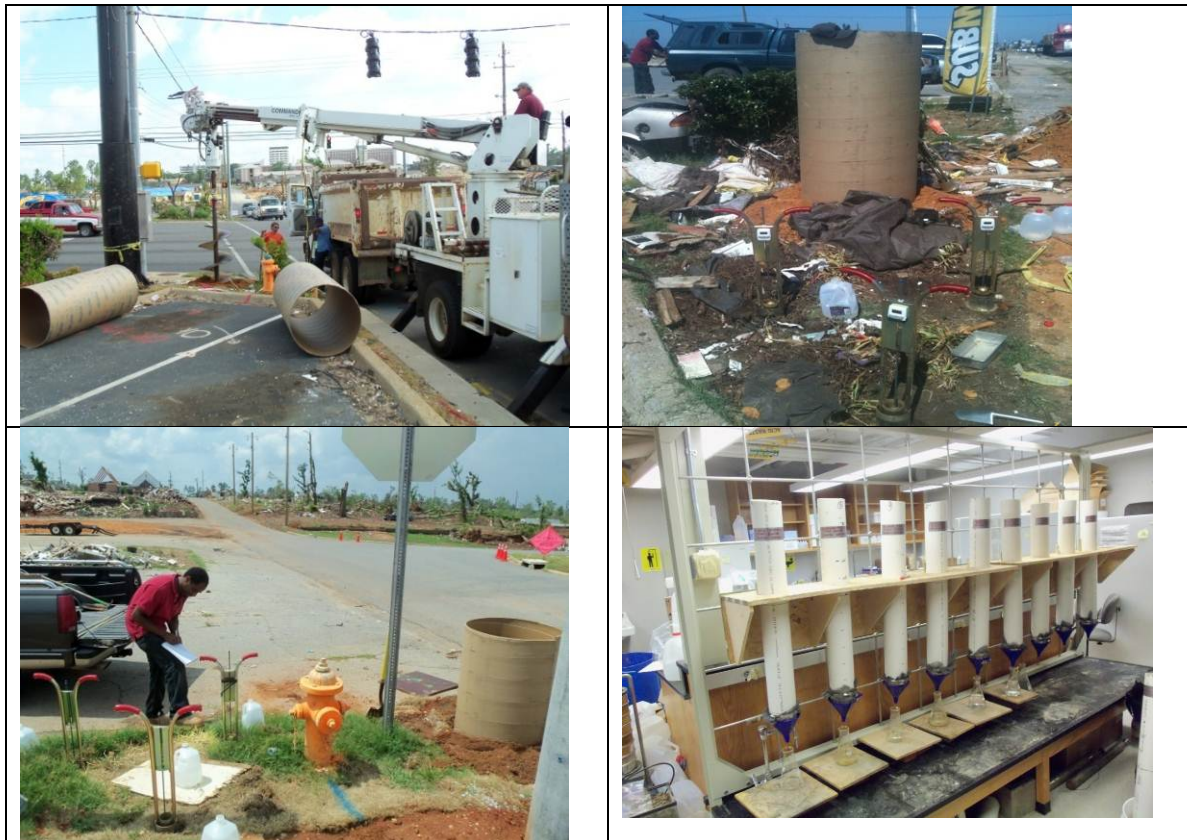
Figure 3. Photographs showing borehole drilling, Sonotube infiltration tube installation, double-ring infiltration measurements, and laboratory column tests.
