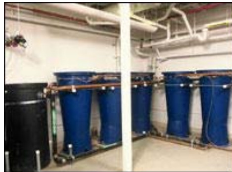
Figure 3-13. NRDC Santa Monica Building's Gray-Water System (Photo: http://www.documents.dgs.ca.gov/bsc/Newsletter/Fall2010/NRDC.pdf )
