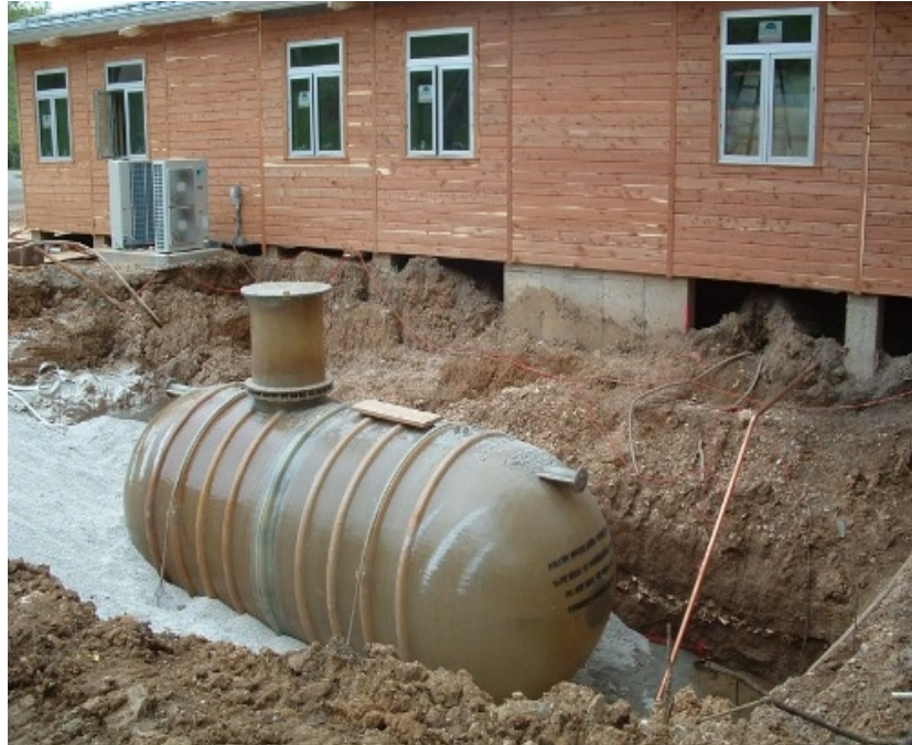
Figure 3-15. A cistern is pictured alongside the Tyson Living Learning Center before being placed underground at Washington University in St. Louis, Missouri ( http://www.solaripedia.com/13/275/2954/tyson_living_learning_center_cistern.html ). (Used by permission of Washington University ©2010)
