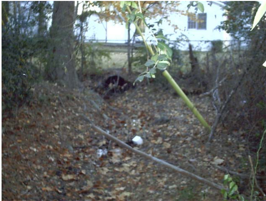
Figure 4.20. Pipe from Insurance Firm Opening into Ditch Flowing into MH 45.1
