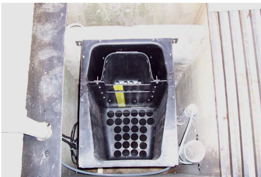
Figure 4.9: Installed prototype UpFlow™ filter (empty) with sampling and monitoring lines
