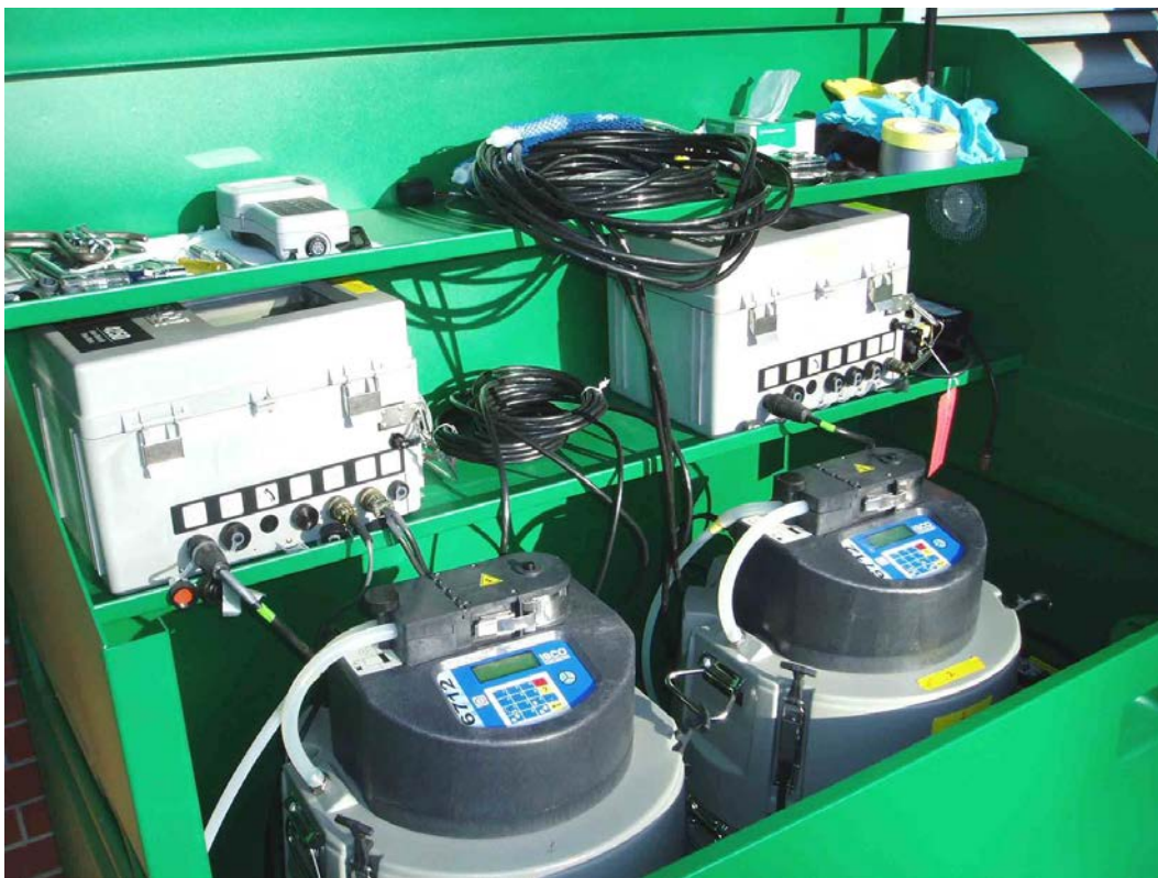
Figure 4.13: Samplers and flow meters in sampling shelter.
