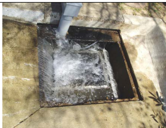
300 gpm showing overflow bypass
