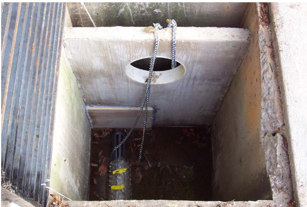
Figure 4.15: YSI Sondes installed in sump (another is behind baffle wall for effluent)
