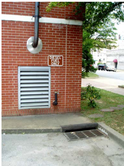
Inlet adjacent to diesel storage area for emergency generator.
