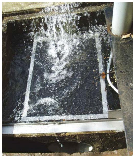
31 gpm flow with Mixed media at capacity
