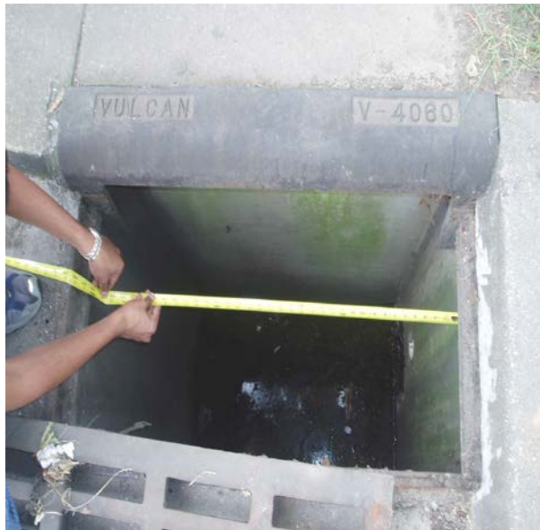
The inlet box is 5 ft deep, 32 inches front to back, and 36 inches wide. The cast cover is only about 18 in front to back, but the city opened it up to full size. The city also installed a baffle wall to separate the inlet into two chambers.
