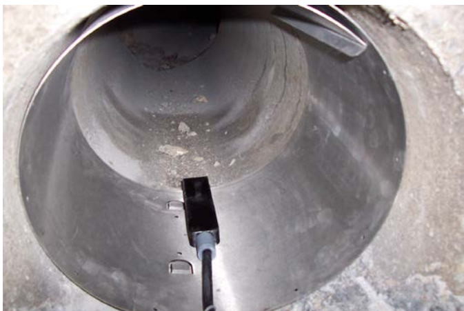
Figure 4.8: Area-velocity sensor installed in effluent pipe.
