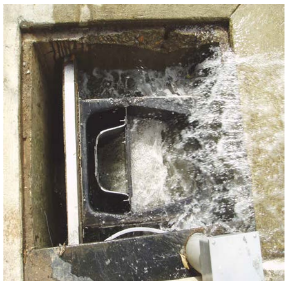
300 gpm into empty chamber with no overflow
