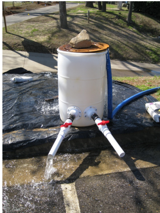
Flow is discharging to the inlet
