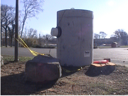
Filter before the installation
