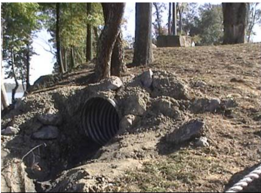
Effluent pipe (before filter installation)
