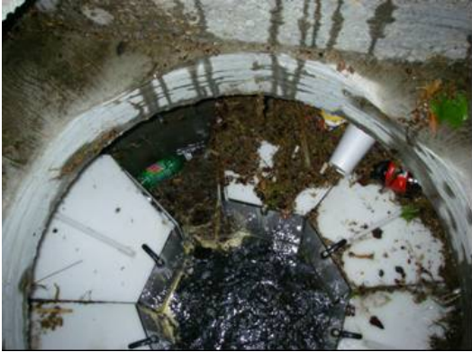
Debris in filter prior to tests
