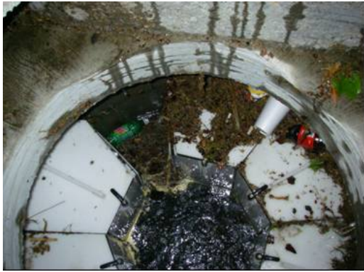
Debris in filter prior to tests
