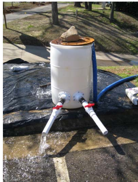
Flow is discharging to the inlet
