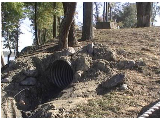
Effluent pipe (before filter installation)
