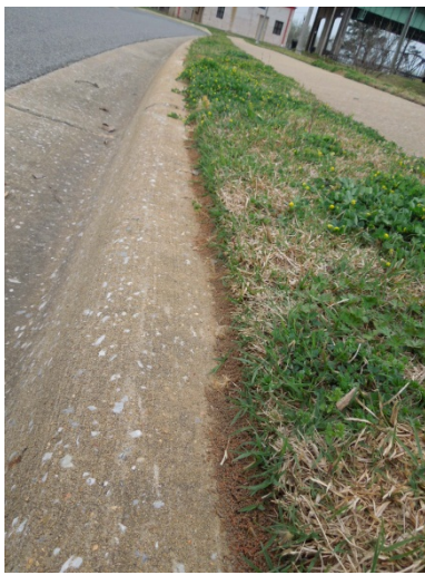
Exposure of some soils beside the roadway due to the activities of ants
