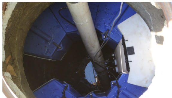
Newly installed roto-molded Up-Flo ® filter modules
