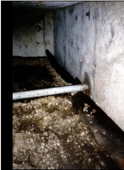
MCTT Filter Chamber At Ruby Garage, Showing Filter Fabric for Flow Distribution and Ballast
