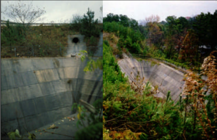
Unusual Dry Detention Pond Located on Hillside to Meet Peak Flow Rate Criterion
