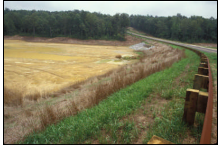
Wet Ponds Located in Areas of Karst Geology may have Sinkholes
