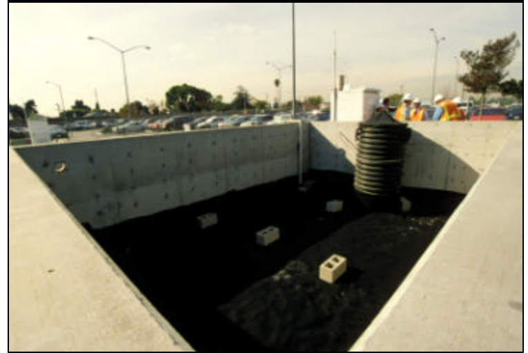
MCTT Filter Chamber at Park and Ride Facility, Los Angeles, CA
