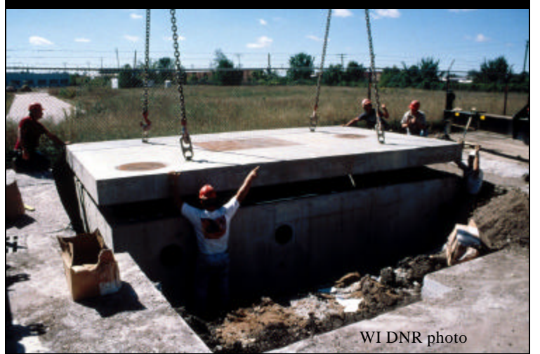
Placing Lid on MCTT at Ruby Garage Public Works Yard, Milwaukee, WI
