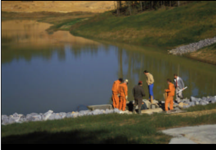
Frequent Maintenance and Adjustments to Outlets may be Needed
