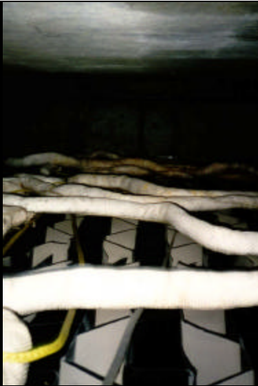
Main Settling Chamber At Ruby Garage MCTT, Sorbent Pillows and Inclined Tubes
