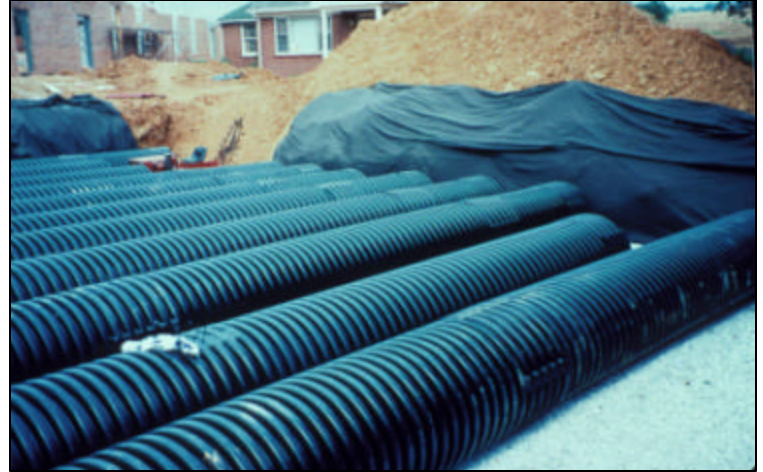
Large Corrugated Pipes used for Underground Detention Below Parking Area
