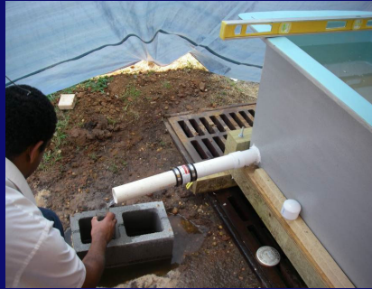
Flow rate measurement from effluent of the biofilter
