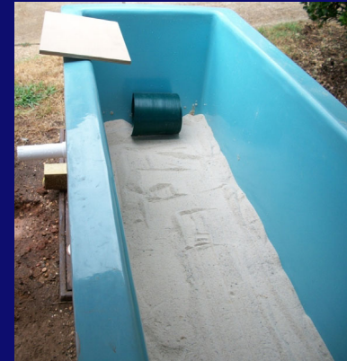
SmartDrain™ installation in the drainage sand (it was unrolled before placement of the cover sand).
