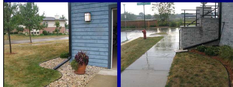
Disconnected roof drain
