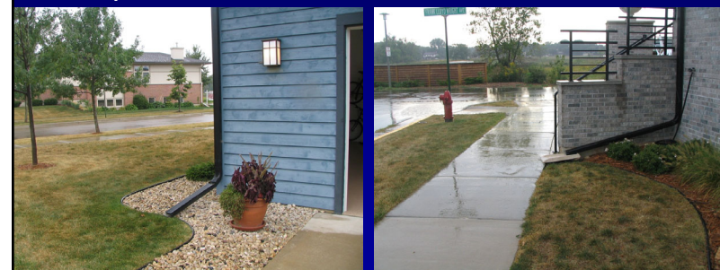
Disconnected roof drain
