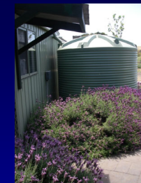
Large water storage tank at Heathcote, Australia winery.
