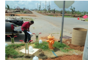
Bore Hole Drilling, Double-ring and Bore Hole Infiltration Measurement Installations (Intersection of 21st Ave. E. and University Blvd E).
