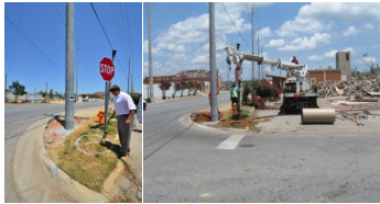
Bore Hole Drilling, Double-ring and Bore Hole Infiltration Measurement Installations (Intersection of 21st Ave. E. and University Blvd E).
