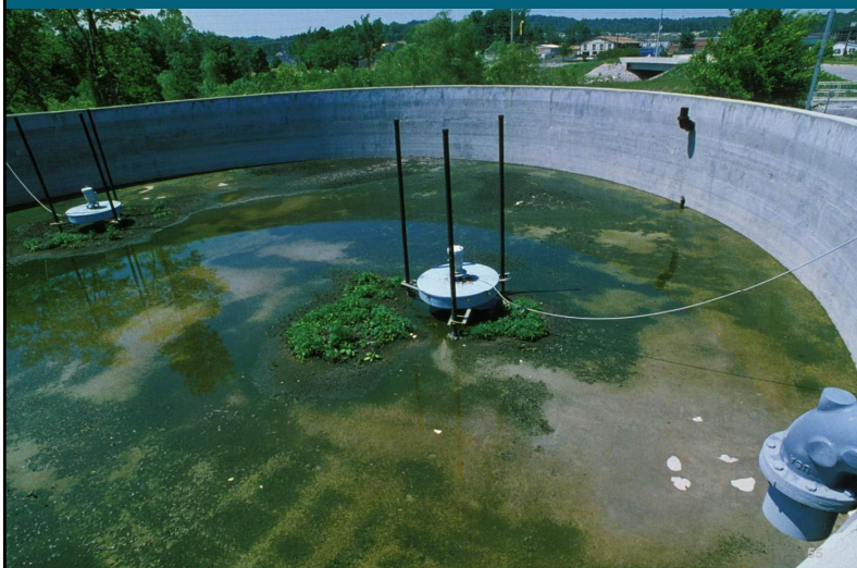
Equalizing Dry Pond to Control SSO Problems, Moody, AL
