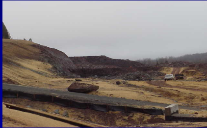
Excavated slopes in the project area. This material is taken to the waste area (D. Lake photo)
