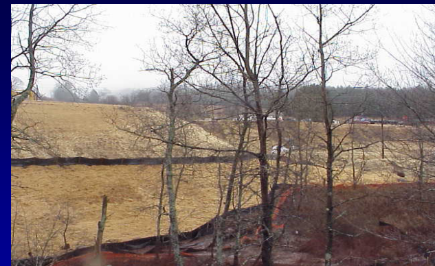
North facing fill slope just south of the Parksville project offices (D. Lake photo)
