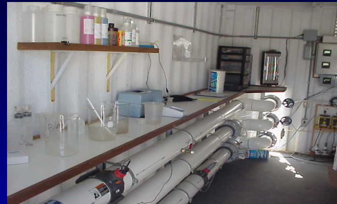
Control center for the polymer operation. Constant monitoring of the NTU levels is provided by the continuous turbidity meters on the back wall (D. Lake photo)
