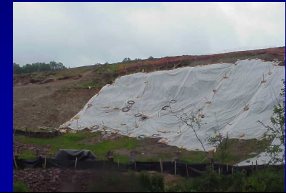
Steep slope at Parksville on-ramp construction covered with plastic to prevent erosion into the Little Beaver Kill (D. Lake photo)
