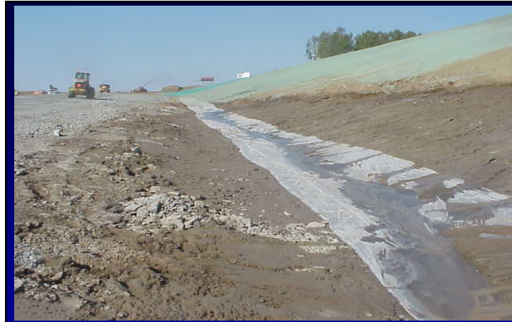
The plastic lined swale conveys groundwater through areas of fine grain soil limiting the erosion. Note the slope stabilization (D. Lake photo)
