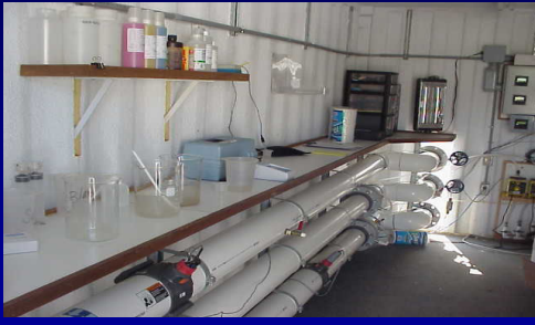
Inside of the control center for polymer injection to sediment pond. Monitoring of the influent and effluent turbidity levels by continuous monitors.
