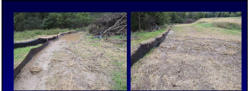
Silt fence and ponding water Material trapped in ponded water area of silt fence
