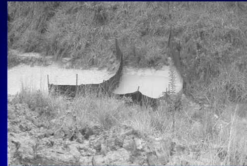
Silt fence check dams on a construction site (practice not commonly approved; silt fences best use for sheet flows)
