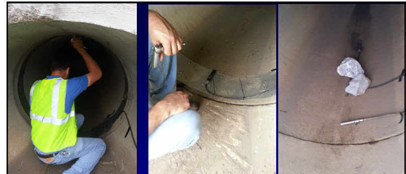
Installation of flow-velocity sensor (and sample intake) into large diameter pipe, and equipment box.
