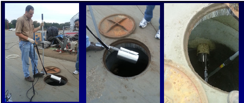
Installation of pipe flume insert, flow sensor, and water sample intake into small diameter pipe.
