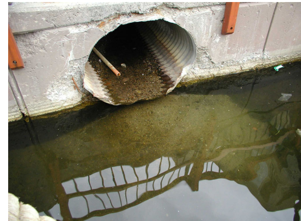
Bedload in corrugated stormdrain and mound of settleable material at discharge into wet detention pond after many years of operation at ski resort at Snowmass, CO (drain from several acre resort parking area having sand applications for traction control).
