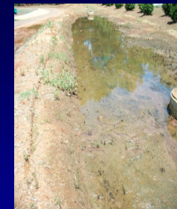
The Vegetation Cover Is Very Poor Indicating Likely Serious Compaction).
