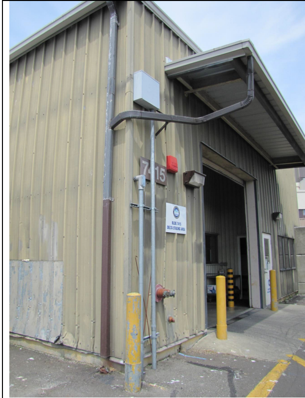
Galvanized metal roofs, painted galvanized w/significant paint peeling of wall. Note broken drainage, connected.
