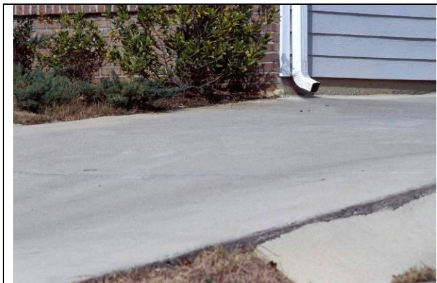
A directly connected roof drain
