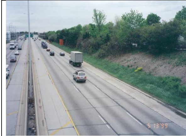
Depressed downtown freeway with eroding embankment
