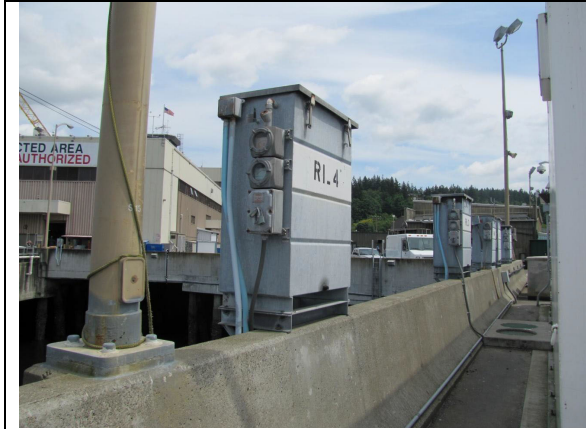
Other galvanized material areas, galvanized utility box, 40 boxes on site at naval base.
