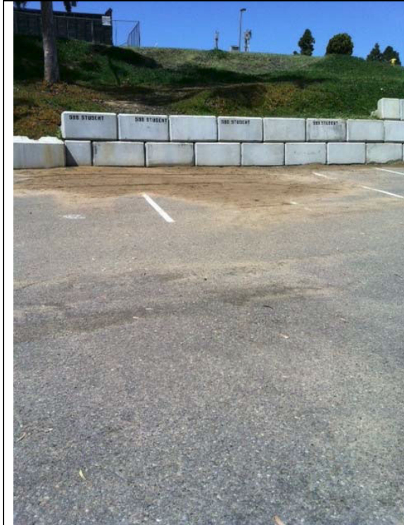
Dirty asphalt parking lot on naval base
