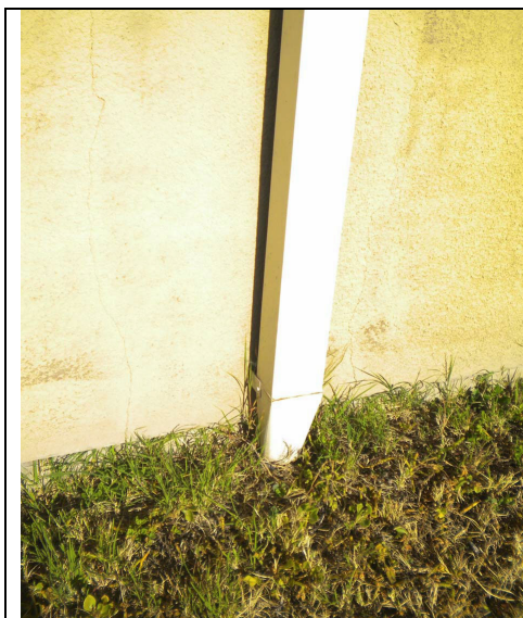
Underground roof drain at navel base (not clear where it is connected)
