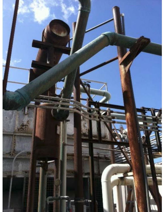
Galvanized and copper piping at naval base
