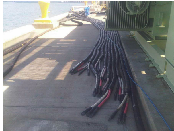
Light laydown area, electrical cables, (on concrete) at naval base
