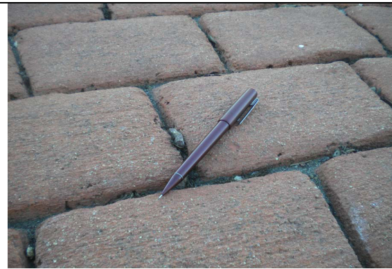
Paver blocks (appear to be grouted so don't allow infiltration, but substantial detention storage during smaller rains) at navel base.
