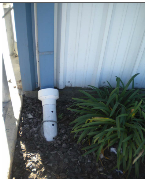
“Underground” roof drain at naval base (showing perforations to allow release if water backs up, possibly draining to underground dry well or french drain)
