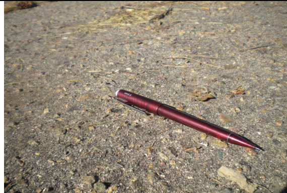
Very rough pavement (worn) at naval base
