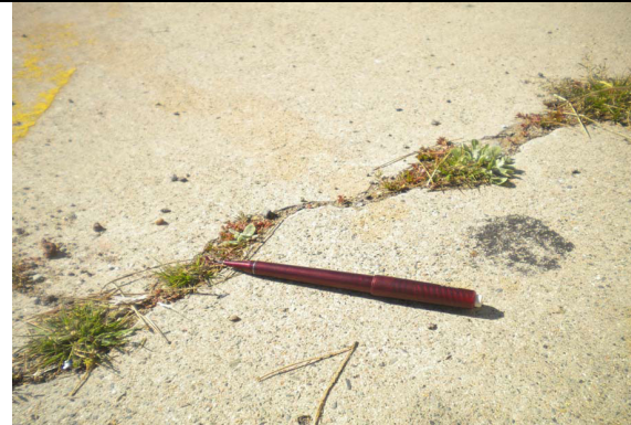
Concrete in poor condition (large numbers of large cracks) at naval base
