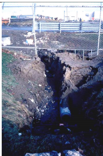
Scoured drain pathway from paved area.
