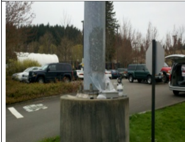
Utility pole, galvanized; NB Kitsap
