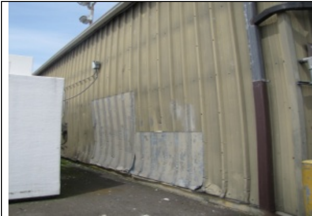
Galvanize siding, painted, chipped; NBK Bangor
