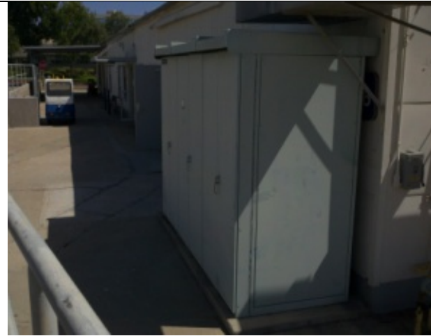
Electrical vault, green; SSC-PAC
