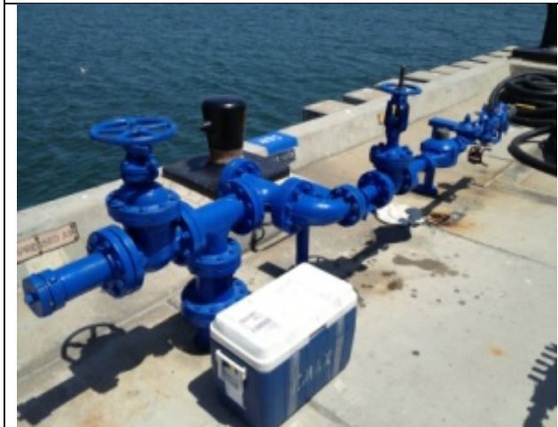
Water riser, potable, blue (w/brass part); Pt. Loma Subase
