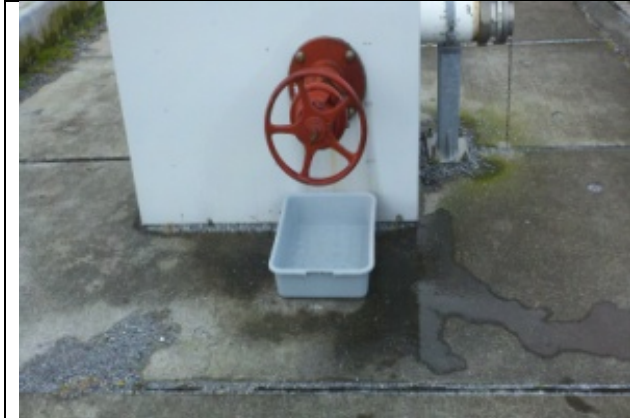
Fire hydrant, red; Everett
