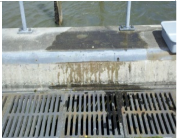
Sheath, over concrete barrier edge; Everett
