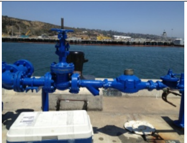
Water riser, potable, blue; Pt. Loma Subase
