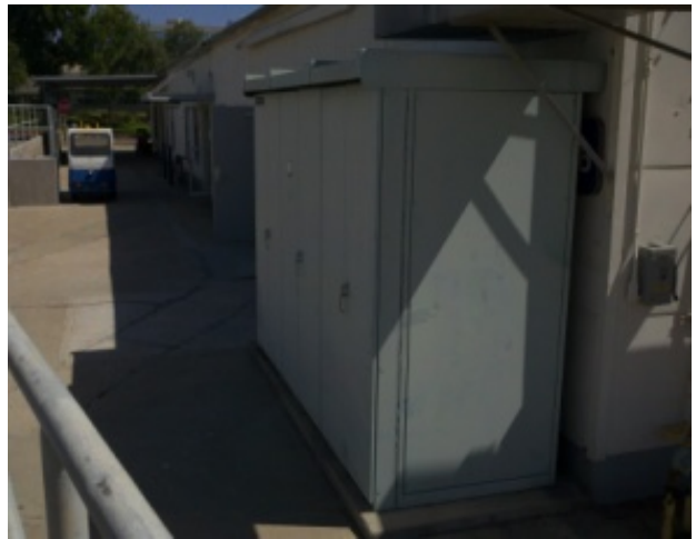
Figure 20: Electrical vault, green
