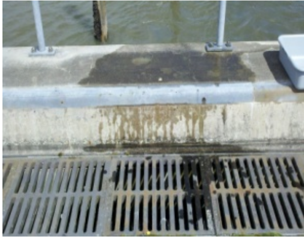
Figure 29: Galvanized sheath, concrete berm
