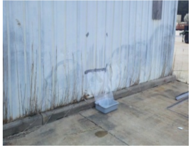
Figure 38: Metal paint, painted, galvanized, building side
