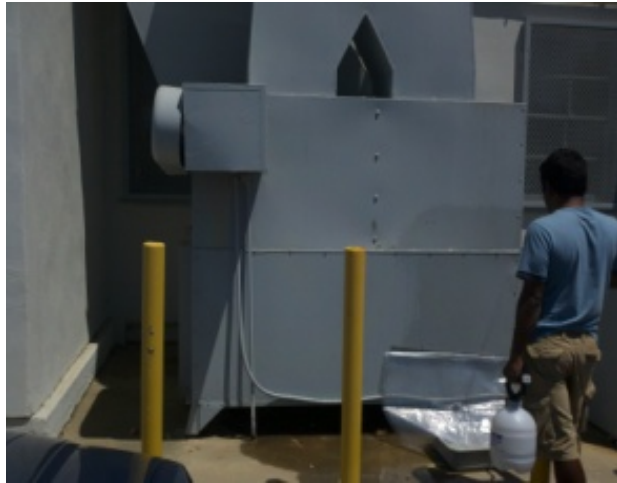
Figure 1: Air conditioning panel
