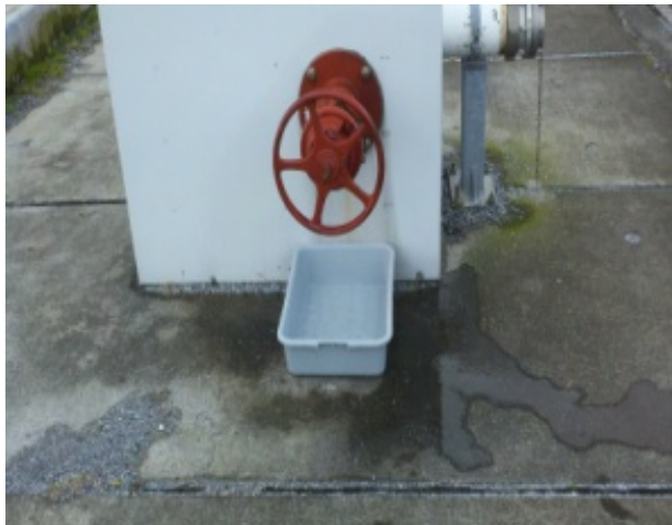
Figure 23: Fire hydrant, red
