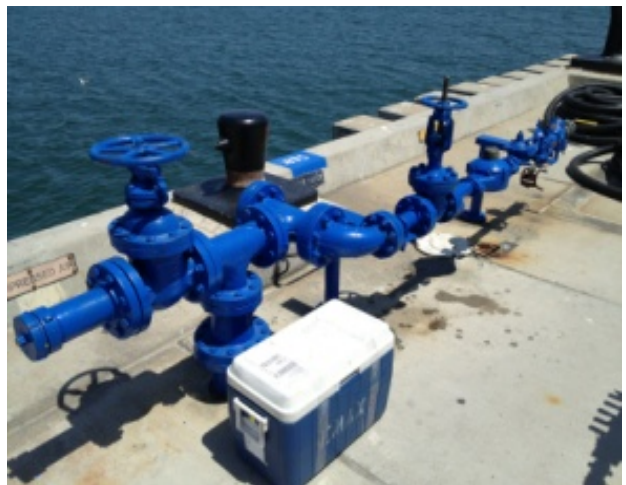
Figure 56: Water riser, potable, blue
