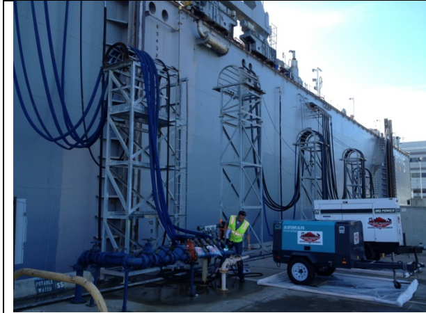
ARCO utility cable racks
