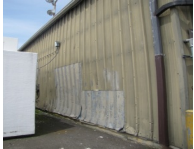
Figure 30: Galvanized panel, painted, chipped
