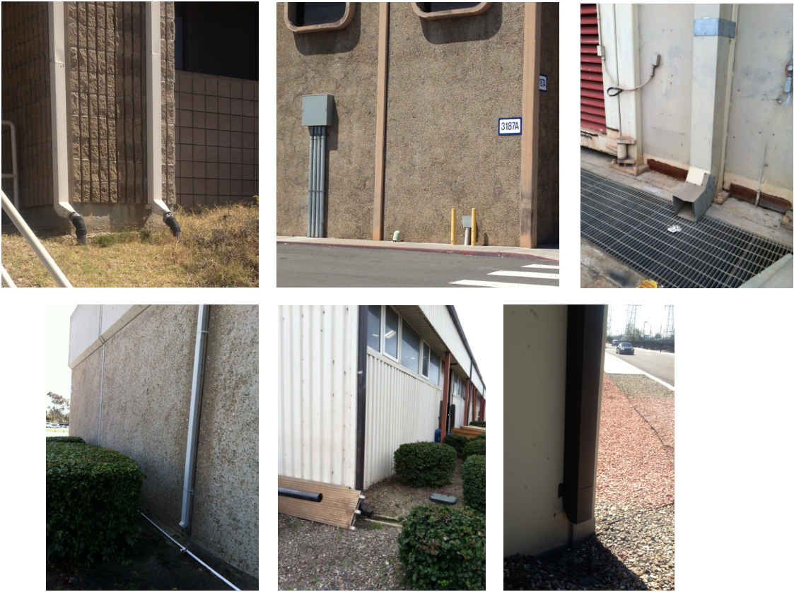
Figure 8. Examples of roofs directly connected to the storm-water conveyance system (top) and those disconnected that drain to vegetation, soil, or stone-filled infiltration areas like those shown in the bottom photos.
