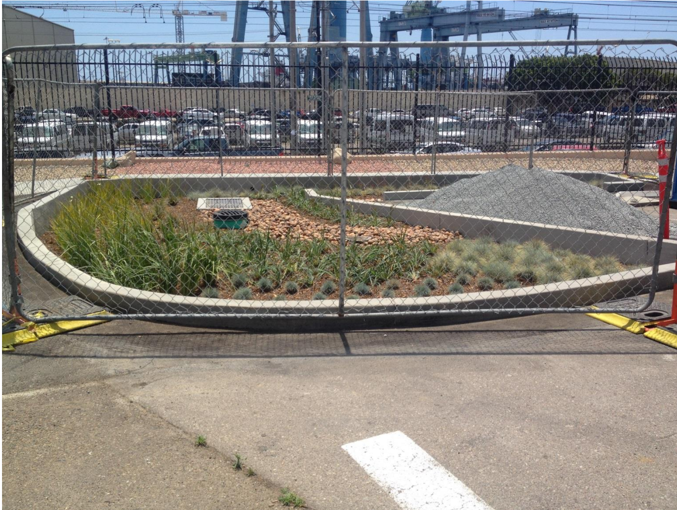
Figure 14. View of nearly completed Biofiltration site facing west. The fencing and extra stone were removed shortly after the photo was taken.
