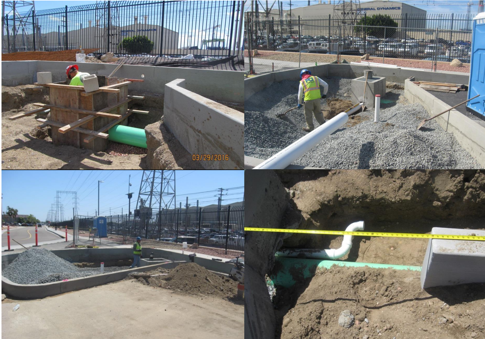
Figure 13. Photos showing various stages of construction of the permeable paver LID technology behind the Commissary.
