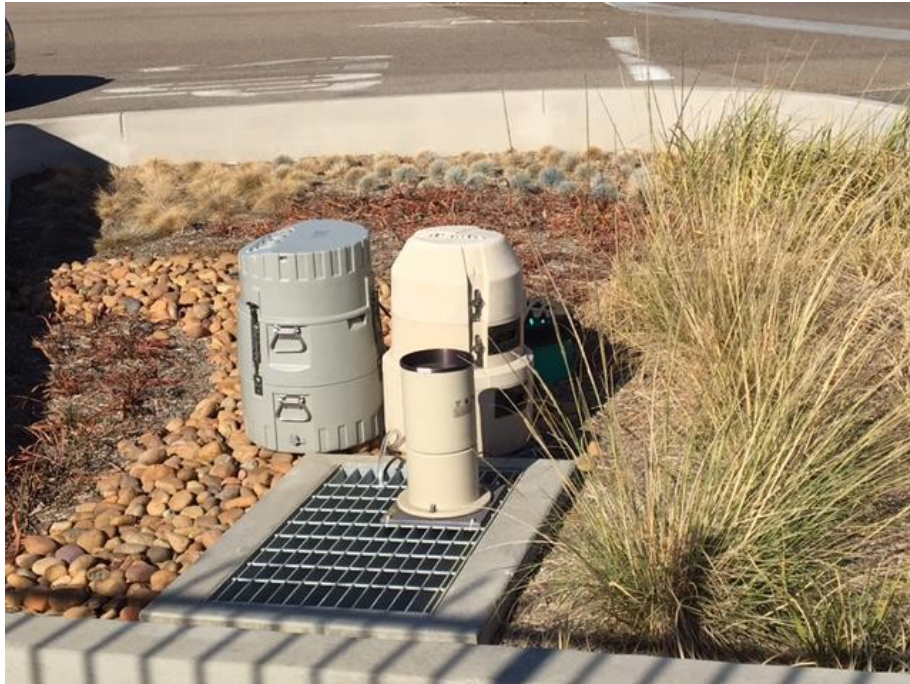
Figure 16. One Teledyne/ISCO and one Hach/ America Sigma stormwater auto sampler set up inside the biofiltration site. One sampler was used to measure stormwater out of the biofiltration underdrain while the other was used measure stormwater draining from the adjacent upstream reference area. The rain gage is shown on top of the vault inlet drain.
