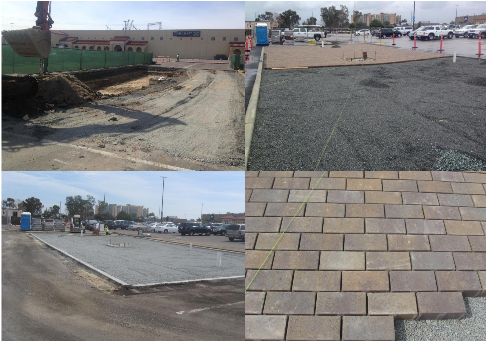
Figure 10. Photos showing various stages of construction of the permeable paver LID technology in front of the Commissary.
