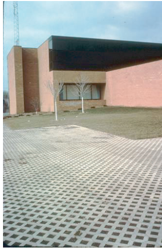
Figure 3.15 Paver blocks for emergency and utility vehicle access, Madison, WI (under construction).
