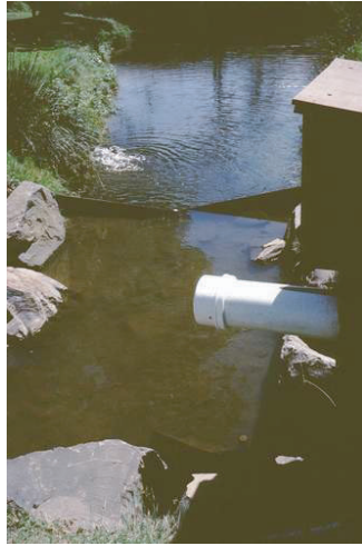
Figure 4.19 Stilling well at Bellevue flow monitoring station.
