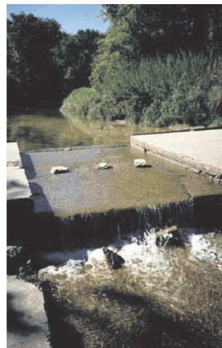
Figure 3.10 Small drop structure obstruction in Lincoln Creek, Milwaukee, WI.
