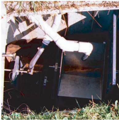
Figure 6.40 Picture of the tipping bucket installation for monitoring surface runoff and subsurface flows at the University of Washington.
