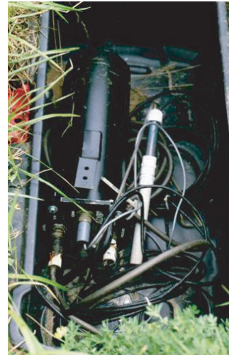
Figure 6.16 ADS acoustic flowmeter at USGS test site.
