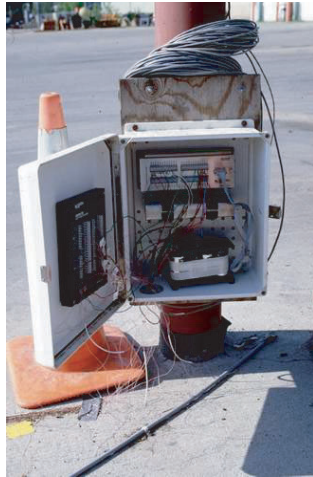
Figure 6.57 Pavement temperature data loggers used by WI DNR.
