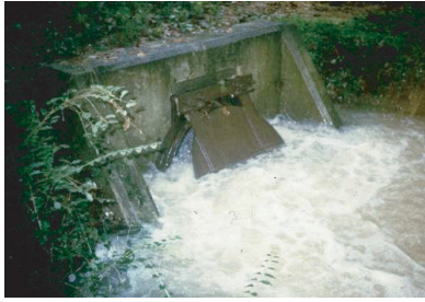
Figure 4.44 Five-Mile Creek SSO discharge during large flow.
