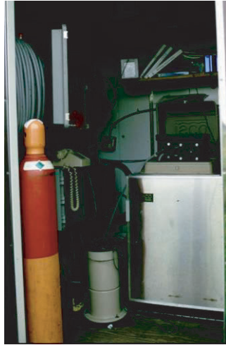
Figure 5.20 Refrigerated automatic sampler in Madison, WI, instrument shelter.
