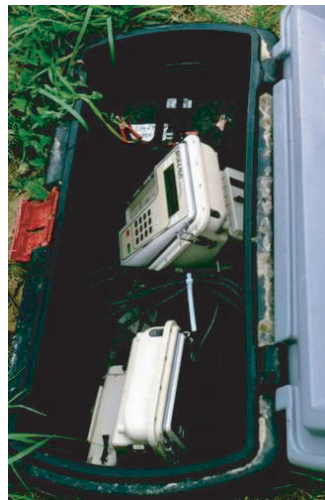
Figure 6.15 Sigma bubbler flowmeter at USGS test site.
