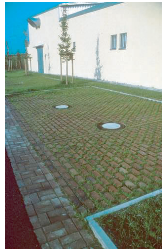
Figure 3.14 Paver blocks for on-site infiltration in Essen, Germany.
