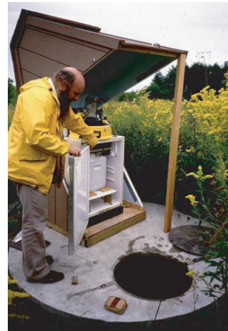
Figure 5.19 Refrigerated automatic sampler located at detention pond outfall in Madison, WI.
