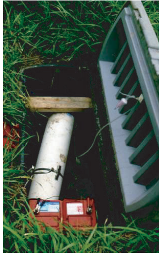
Figure 6.17 Acoustic flowmeter at USGS test site.
