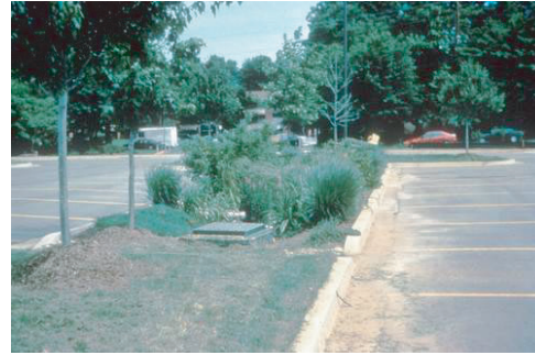
Figure 3.20 Biofiltration in parking area (Photo used with permission of Center for Watershed Protection.)
