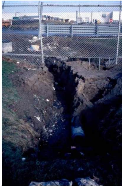
Scoured drain from paved area.
