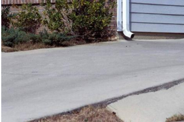
A directly connected roof drain
