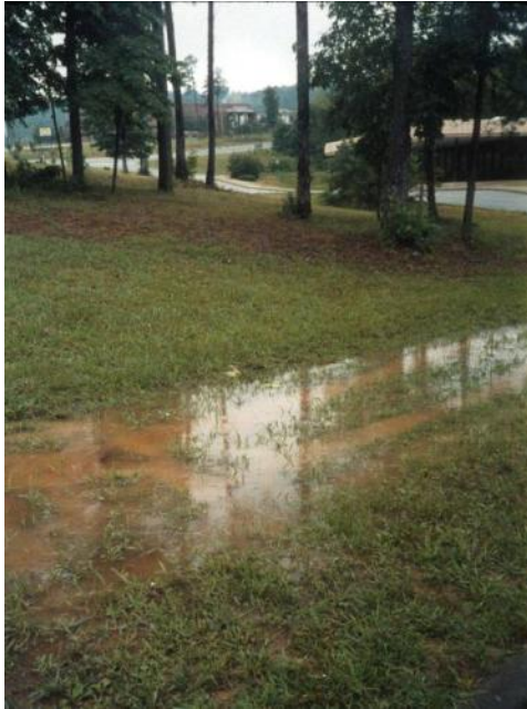
Soil erosion from landscaped areas having fine-grained soils during periods of high rain intensities
