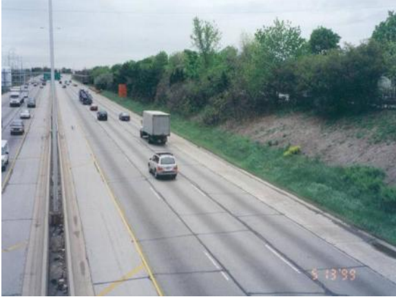
Depressed downtown freeway with eroding embankment
