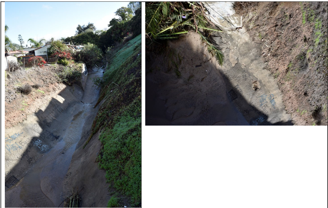
Figure 18. Paleta Creek near Solola Ave. and Euclid Ave. showing potential erosion sources.
